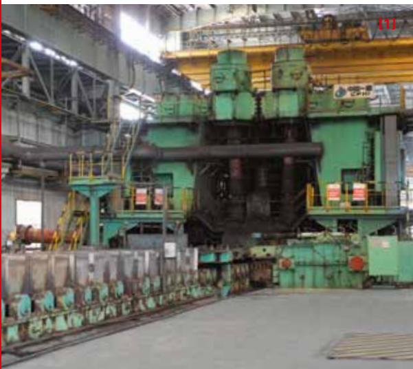
[1] | Rougher with edging stand. [2] | Steckel rolling mill with cooling system.
